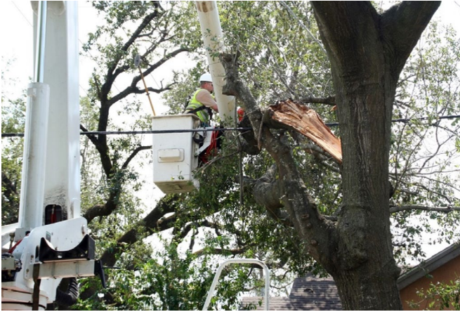
Figure 6. A utility arborist removes a conflicting tree that has broken in a storm and damaged utility lines. (Photo by Greg Henshall, FEMA, via picryl.com.)
