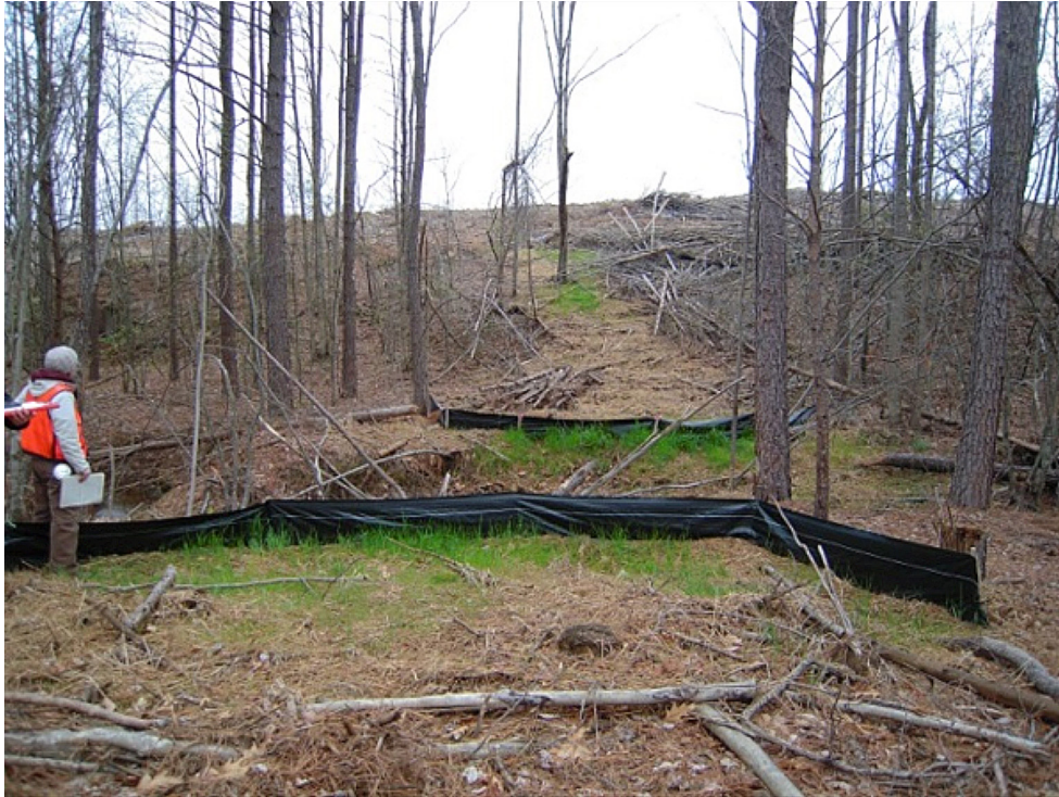
Figure 4. Temporary crossing closure with “mulch + silt fence” (water bars, seed, lime, fertilizer, straw mulch, and silt fence at stream).
