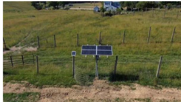
Figure 12. Photo of a 400W PV Array for a Solar Water Pumping System
