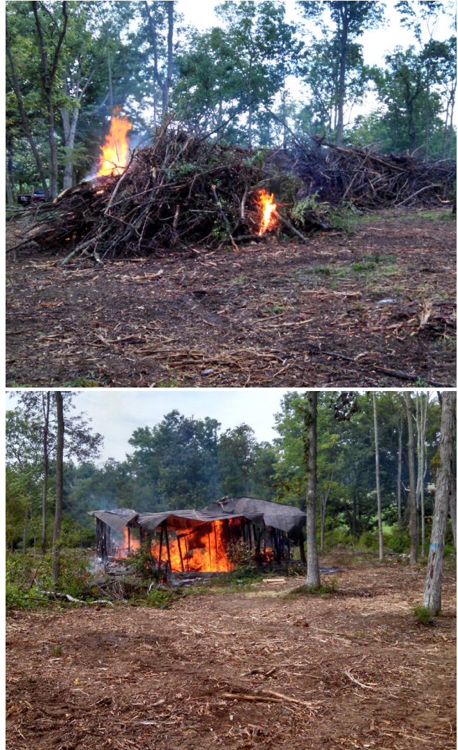
Figure 6. Mulching and burning (including an old homestead, bottom) were needed to clean up this demonstration site at Steeles Tavern. “Leave” trees were first marked before thinning operations, and the residual materials were mulched or piled and burned. In this instance, the large piles of residuals represented a cost to pile up and burn, and some of its nutrients were lost; in some cases, the fire also was too close to trees and caused damage to the tree stand. A preharvest mulching that removed the invasive understory could have facilitated harvest and reduced the residual cleanup, while the chips would have protected soils during harvest operations. (Photos by Adam Downing.)
