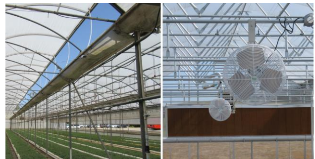
Figure 2. Venting the greenhouse can be via natural airflow using dropdown sides and ridge vents (left) or mechanical by pulling outside air through cellulose water walls (right). (Joyce Latimer, Virginia Cooperative Extension)
