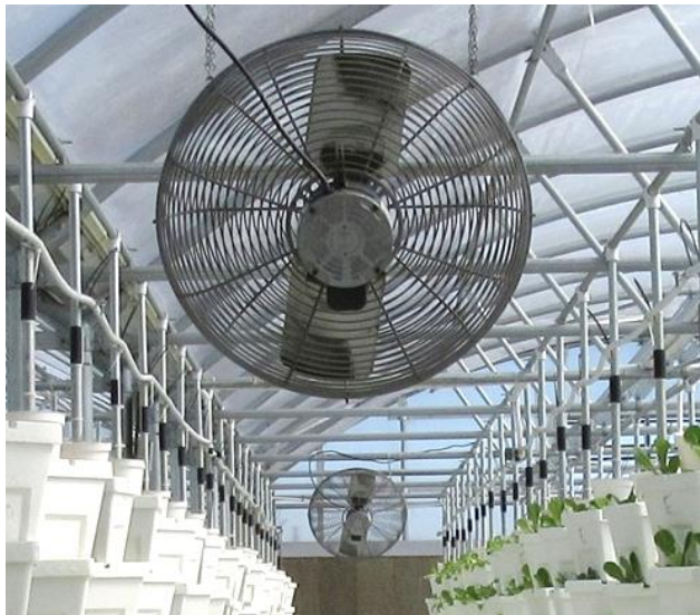
Figure 3. Horizontal airflow fans (HAF) should run whenever the greenhouse is not venting to ensure good air circulation around the plants. (Joyce Latimer, Virginia Cooperative Extension)
